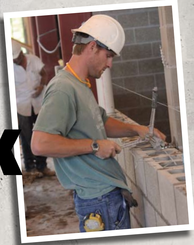
Lake Country Masonry Inc. worker Jared Lystig constructs a wall at the new Northwestern High School in Maple, Wis.
